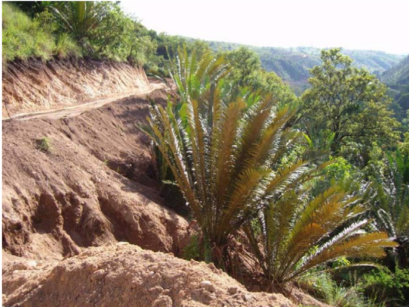
Fig. 6 Deep gully created due to soil erosion after road construction in the cycad belt
